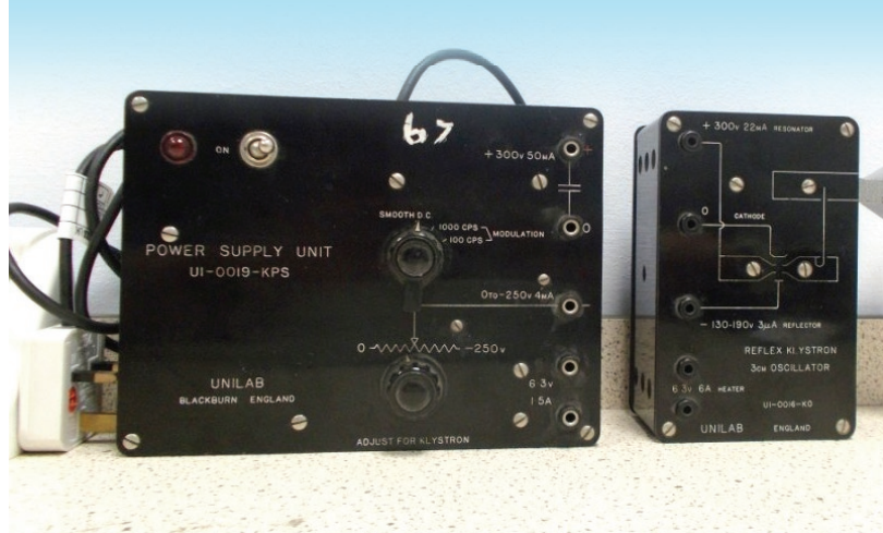
Figure 3 - Potentially dangerous power supply.
